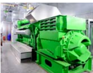
CHP engine protection
