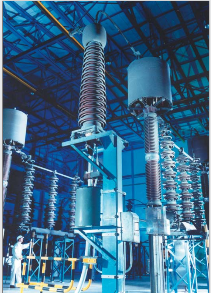
Power station (Peterhead CS)
