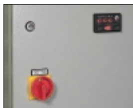
Front view of a cabinet with the display unit, easily visible, mounted on the front of the door, whilst the protector unit is installed deep within.
